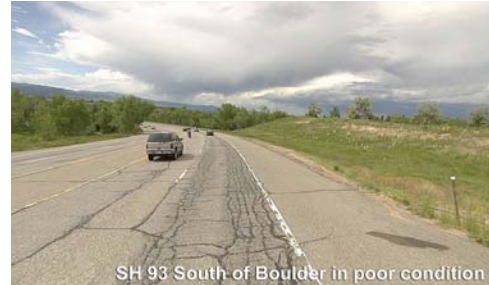
SH 93 South of Boulder in poor condition
